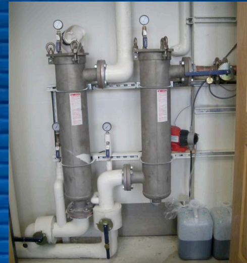
Rainwater Purification Filters
